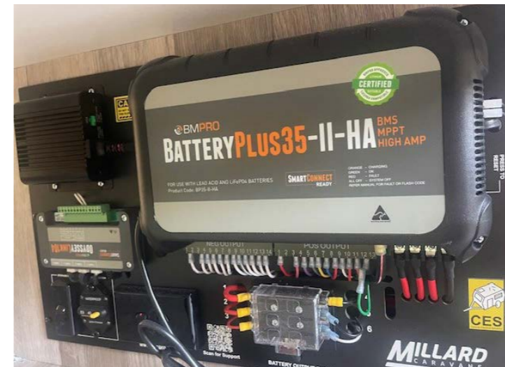
Battery Management System
